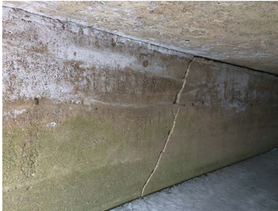
EAST ELEVATION, EAST WALL SEVERE DIAGONAL CRACKING, NORTH CRACK
