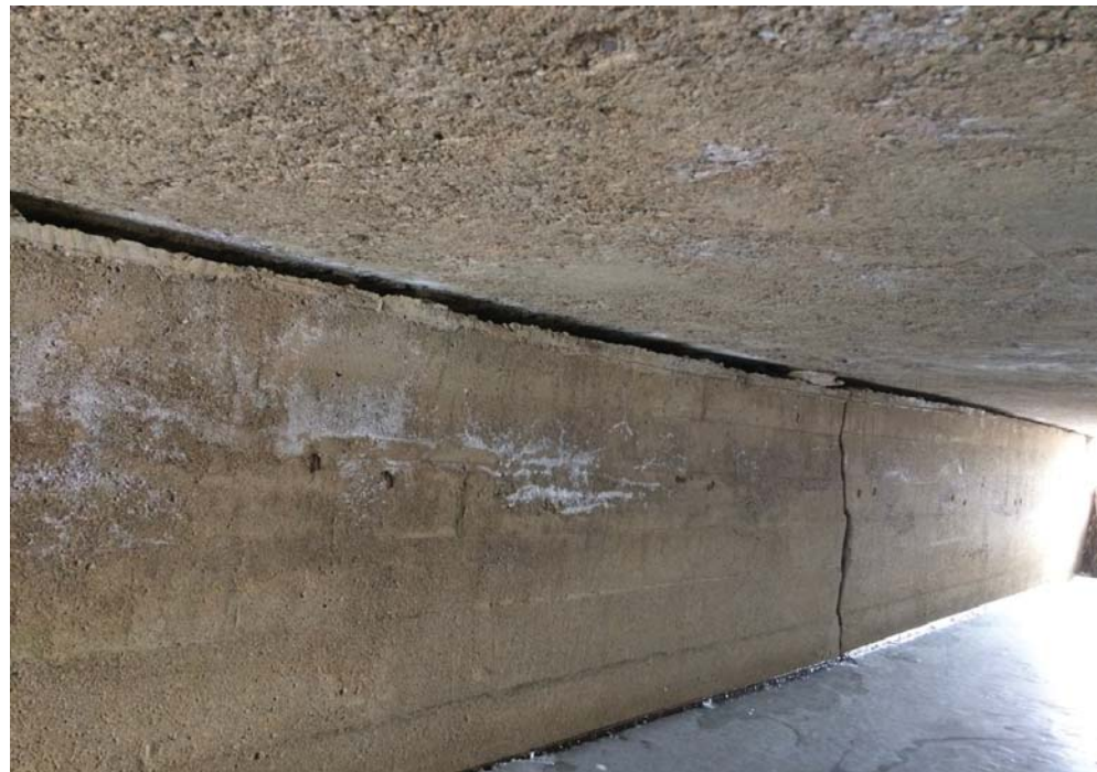
EAST WALL, SOUTH CRACK, AND WALL TO SLAB SEPARATION
