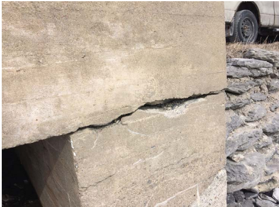
EAST HEADWALL / NORTH WALL, WEST ELEVATION CRACKING AND SEPARATION OF HEADWALL
