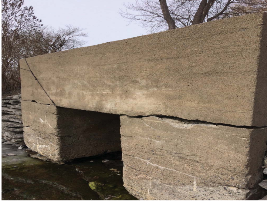
SOUTHWEST ELEVATION SEPARATION OF HEADWALL AND DETERIORATED CONCRETE WALLS
