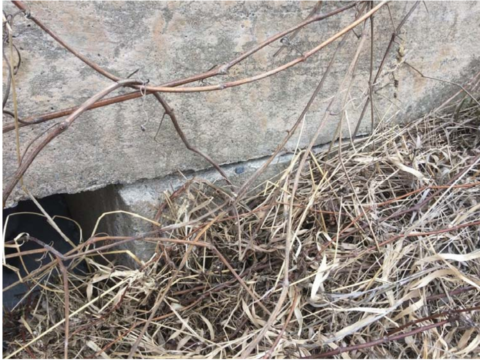
WEST ELEVATION, SOUTHEAST WALL ROOF SLAB TO WALL SEPARTION,
