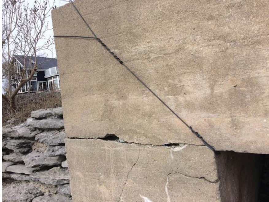
EAST HEADWALL / SOUTH WALL, WEST ELEVATION, CRACKING AND SEPARATION OF HEADWALL
