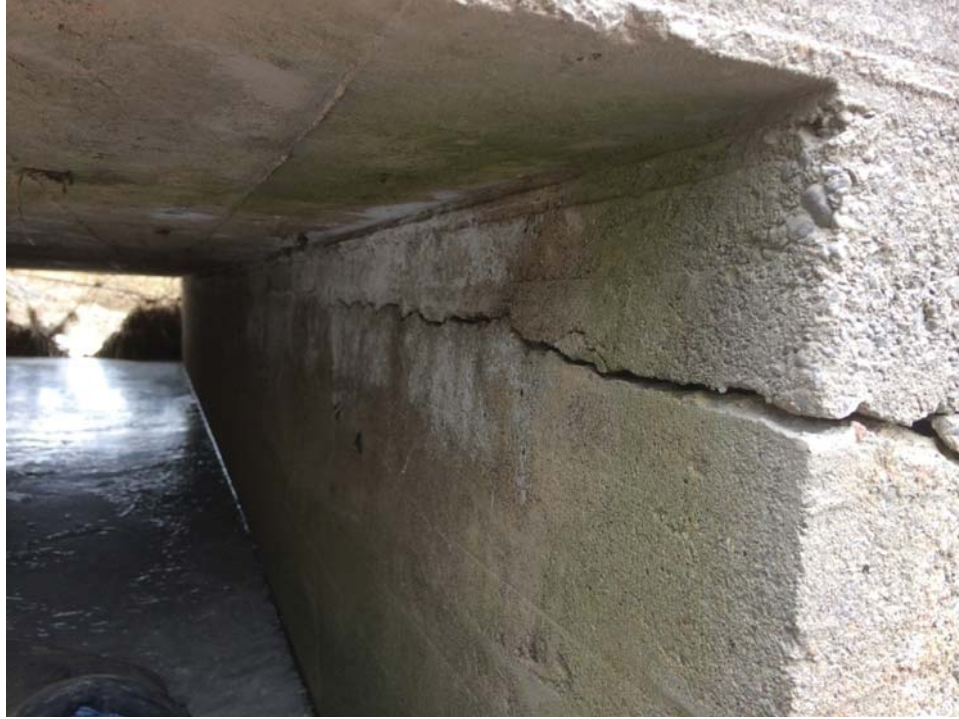
SOUTH WEST ELEVATION, WEST WALL SEVERE CRACKING AND SEPARATION
