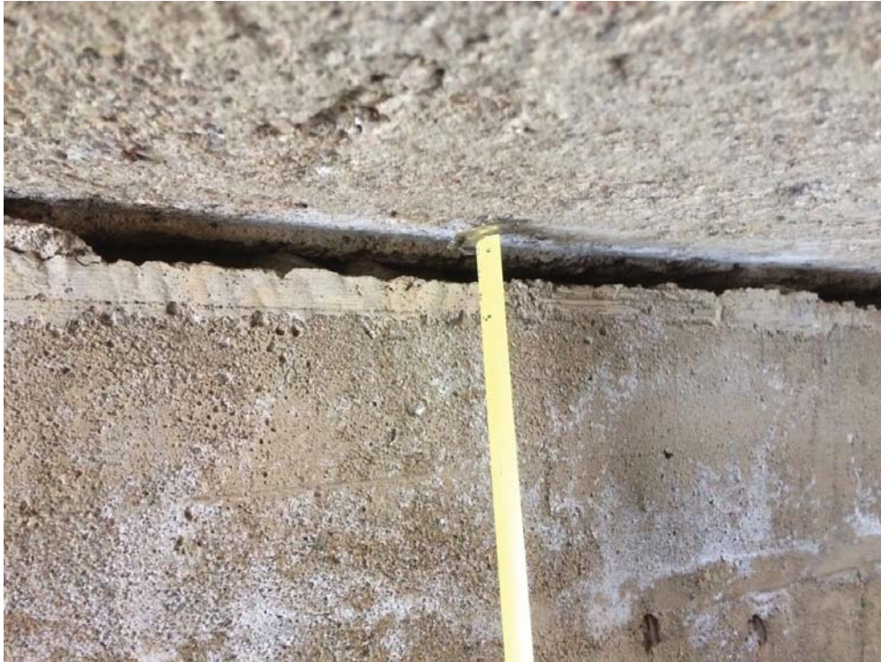
EAST WALL, 25mm ROOF SLAB TO WALL SEPARATION
