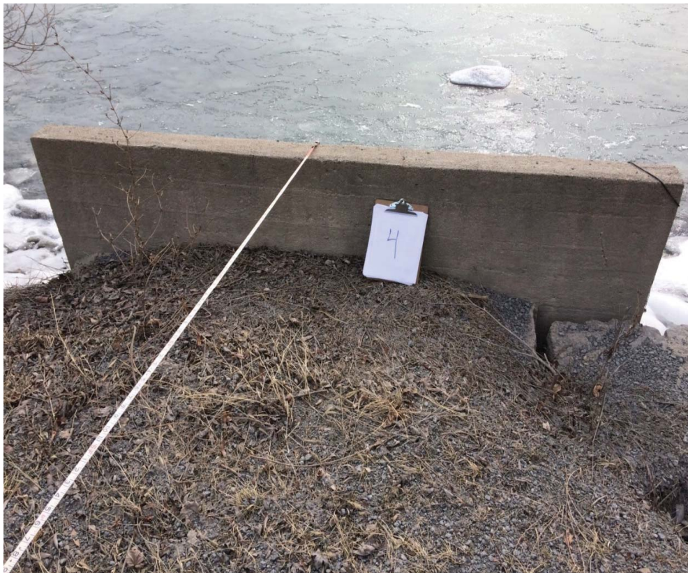
OUTLET LOOKING EAST, CRACKING AND EROSION AT HEADWALL
