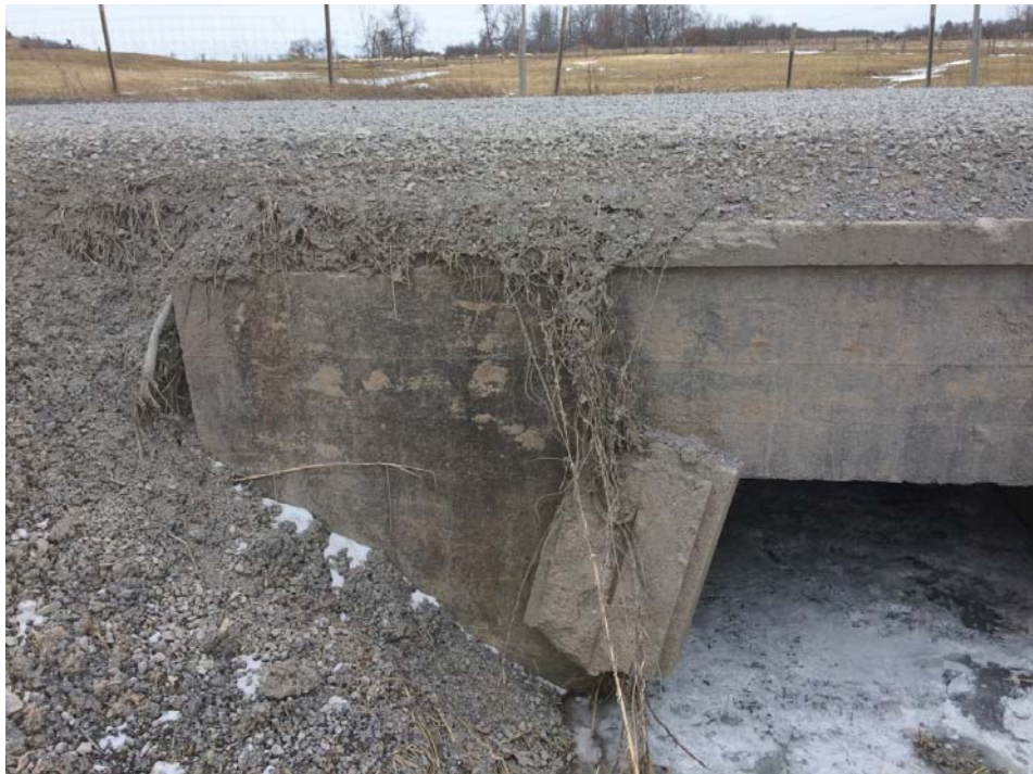
EAST ELEVATION, SOUTHEAST WALL DISINTEGRATION OF SMALL HEADWALL
